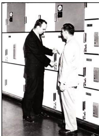
Bob Mathews of Osborne Electric and Newton Johnston of General Electric discuss the FAA Center switchboard in the 1960s.
